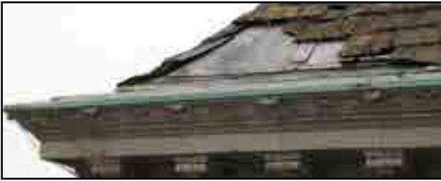
Damage to Collyweston slate
