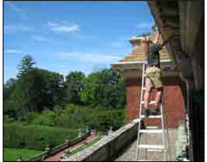
Roof condition is checked by Doreen Lumbr from Old Westbury Gardens' Operations and Maintenance staff
