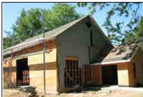
The barn renovation as of early December, far left, and late May, left
